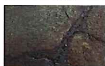
Photo 4: Water penetrating cracks in spillway as observed by residents.
