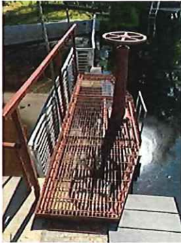
Photo 10: Outlet Pipe Gate Operator
