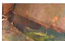
Photo 5: CCTV footage showed the gate does not seal against the concrete structure.
